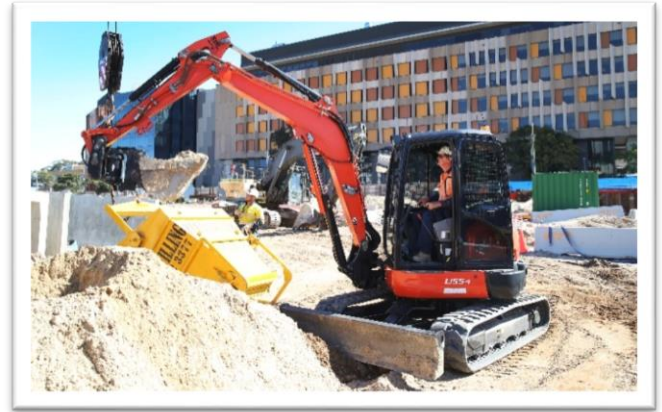
A construction worker backfills trenches as part of important stormwater infrastructure upgrades.
