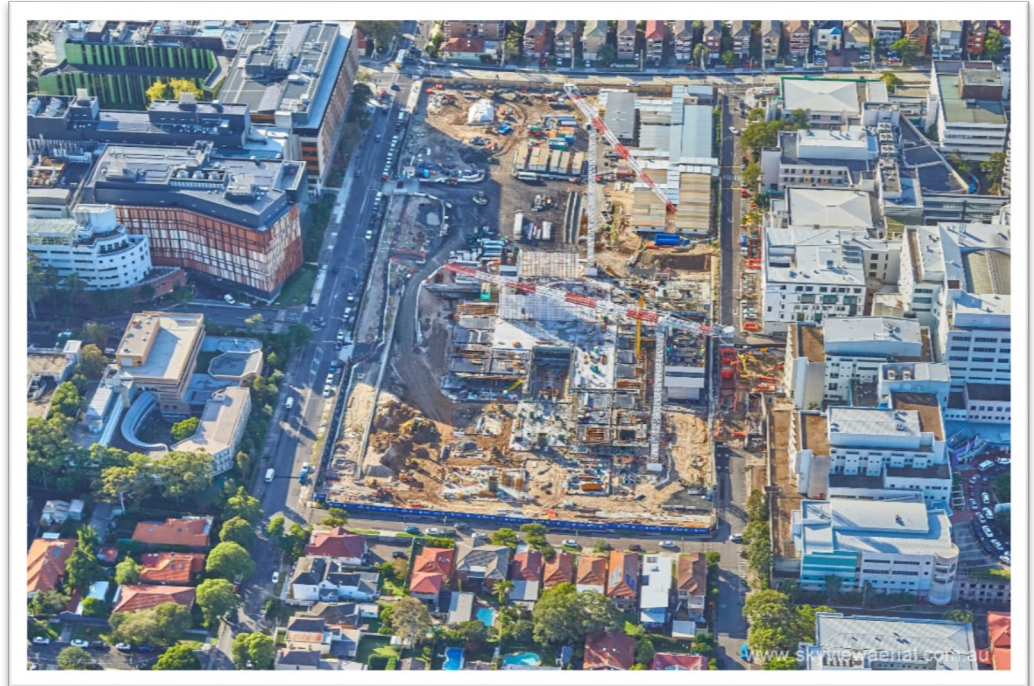
Aerial view of the Randwick Campus Redevelopment construction site showing commencement of main building structural works.
