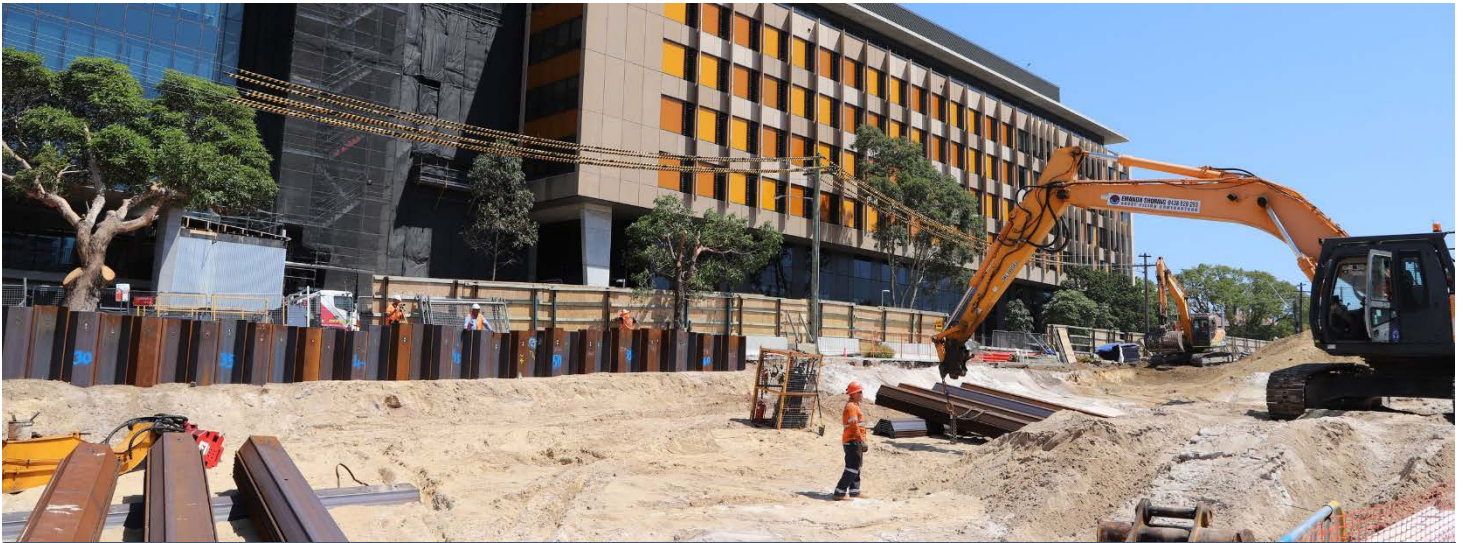
Construction workers install temporary sheet piles to allow work to commence on upgraded stormwater infrastructure along the Botany Street site frontage
