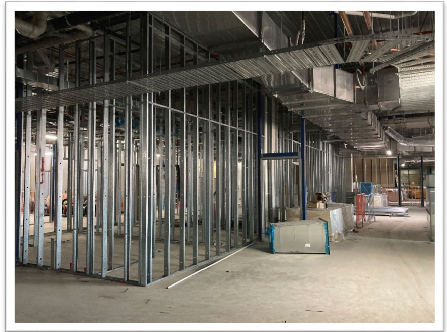
Services installation and fit out continues on the floors of the IASB
