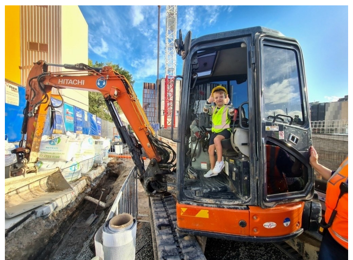
Pictured: Andy on the construction site with his dad; kids take turns sitting in the excavator
