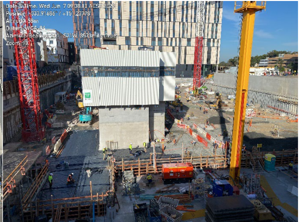
Sealed construction area. Waste receptacles around work site. Plant with identifiers e.g., GRC139 Komatsu plant.
