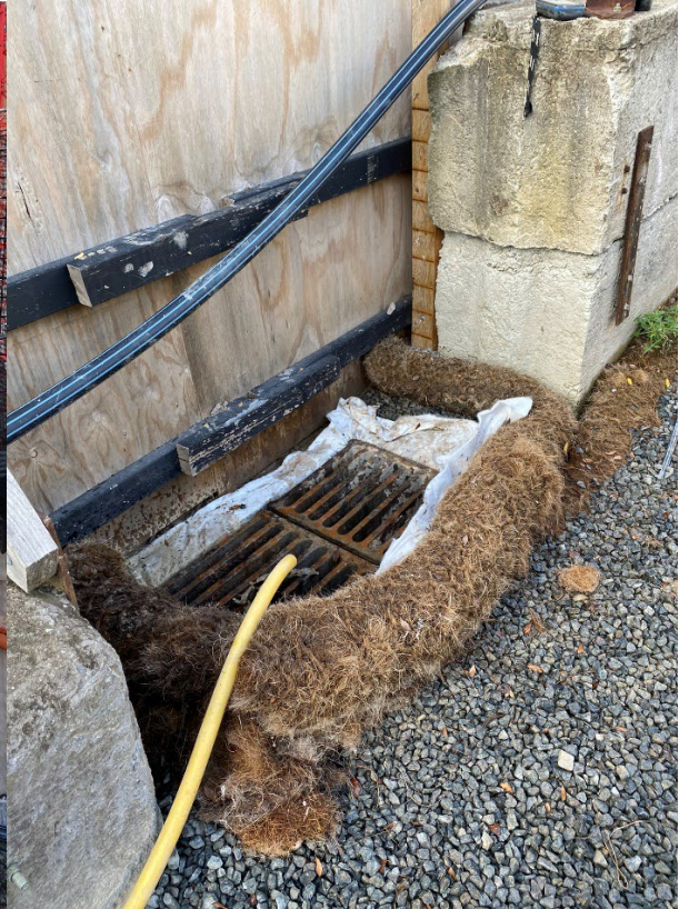
Covered drain surrounded by a coir log along Hospital Road, adjacent to the hoarding.
