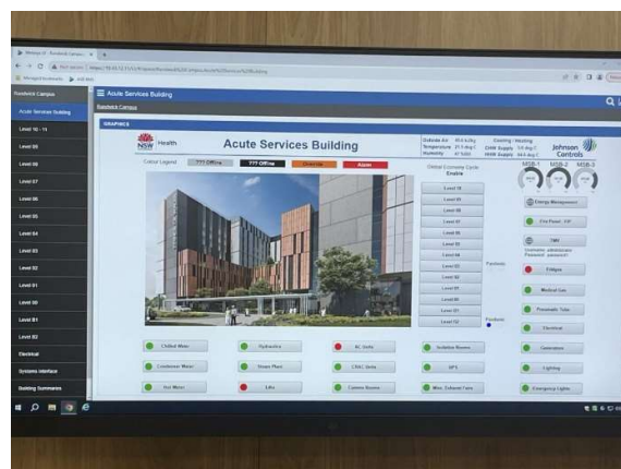
ASB Maintenance System
