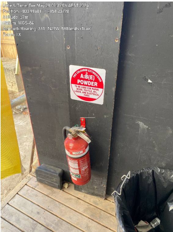
Wall mounted fire extinguisher.
