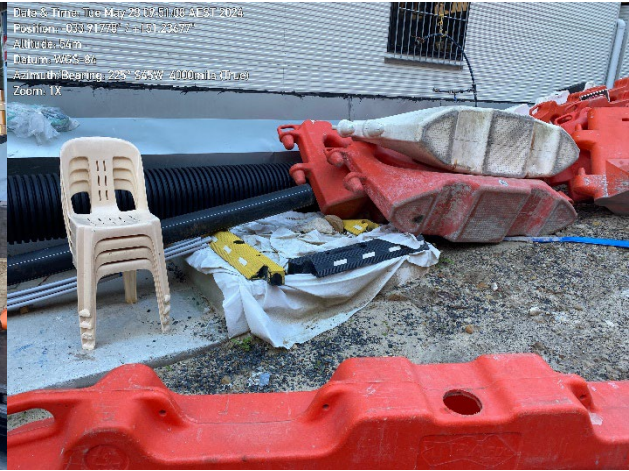
Covered drain surrounded by a coir log adjacent to site temporary driveway from Botany Road.
