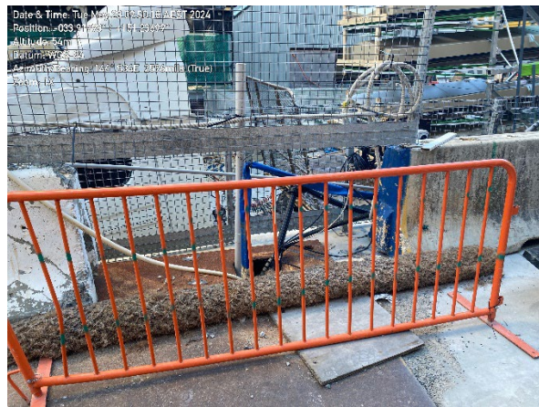
Controls around OSD tank.
