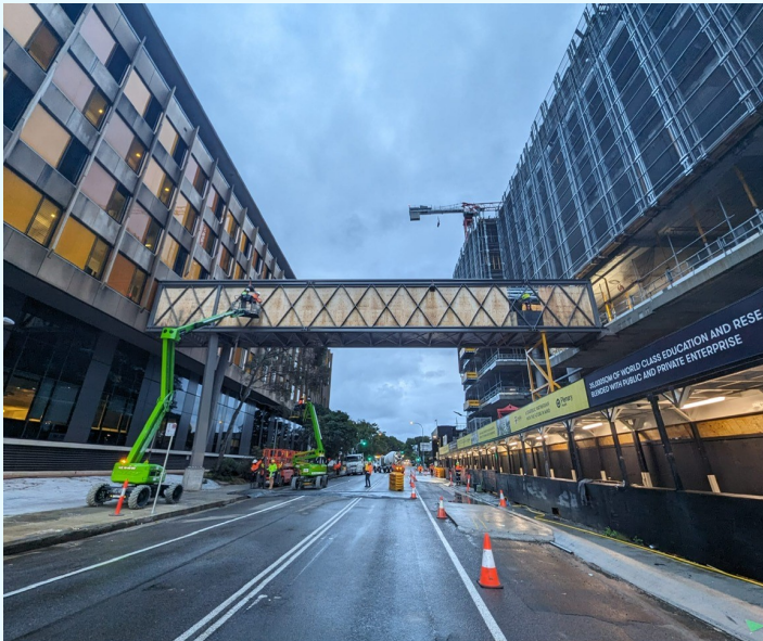
Pictured: The HTH to Wallace Wurth Building pedestrian link bridge over Botany Street, during installation of the structure in 2024.
