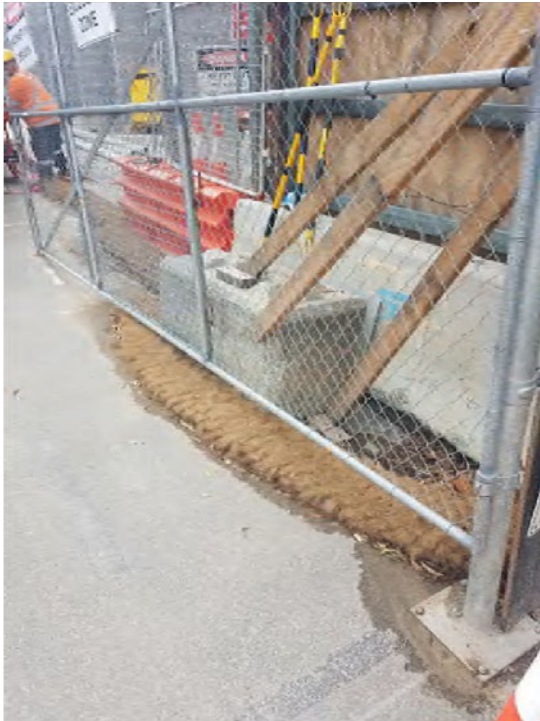
ERSED controls at gate ready to deploy
